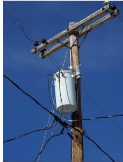
Frank and his crew are inspecting residential transformers Courtesy Wikimediacommons, image is in the public domain
