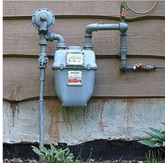
Tom is checking gas meters Courtesy DOE, image is in the public domain
