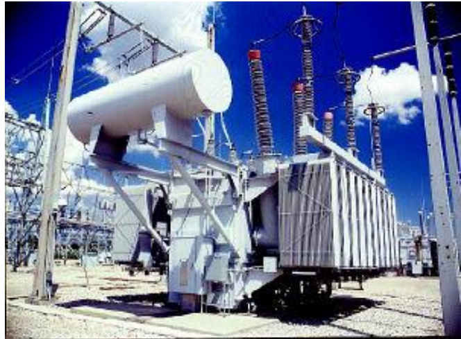
Leala was adding oil to substation transformers Courtesy OSHA, image is in the public domain
